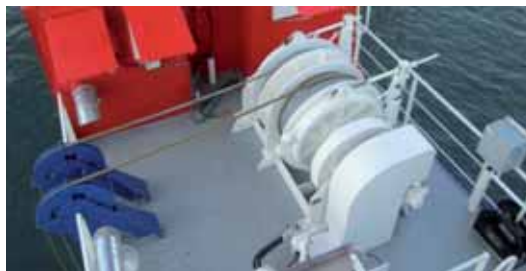
Hydraulic Mooring and Anchor Winches Submersible Pontoon: Kugira II Owner: Acciona / Country: Spain
