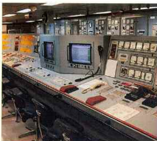
Machine Control Room of a frigate
