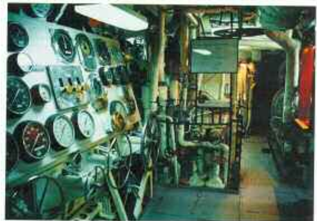
A view of the machine room
