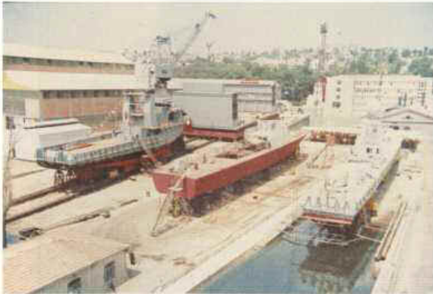
TWO FAST PATROL BOATS, A TUG BOAT AND A FLOATING DOCK PONTOON UNDER CONSTRUCTION
